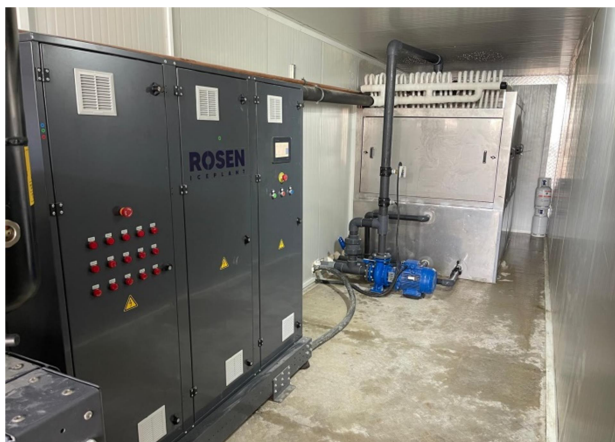
-Evaporator and Control Panel-
