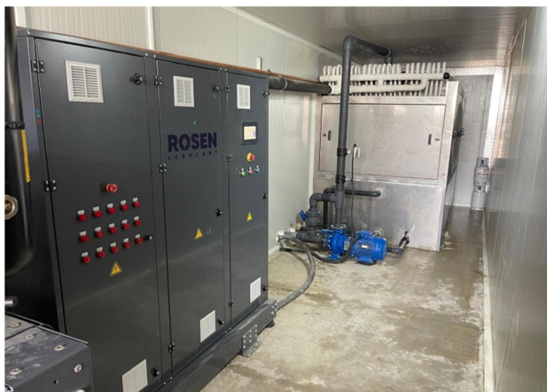
-Evaporator and Control Panel-
