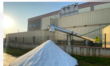
Screw Conveyor for Ice Delivery
